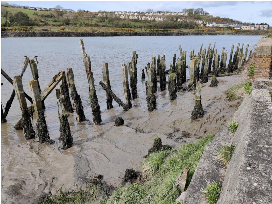
Plate 2.13 The River Suir at Ch. 960, comprising 'Tidal rivers', including 'Sea walls, piers and jetties', 'Lower salt marsh', 'Mud shores' and 'Estuaries'. More detailed photos of these habitats are presented in the Intertidal Survey Report (Brophy, 2021) in Appendix B to this NIS.
