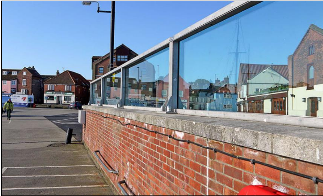
Plate 2.5 Example of a glass flood barrier installed along a wall
